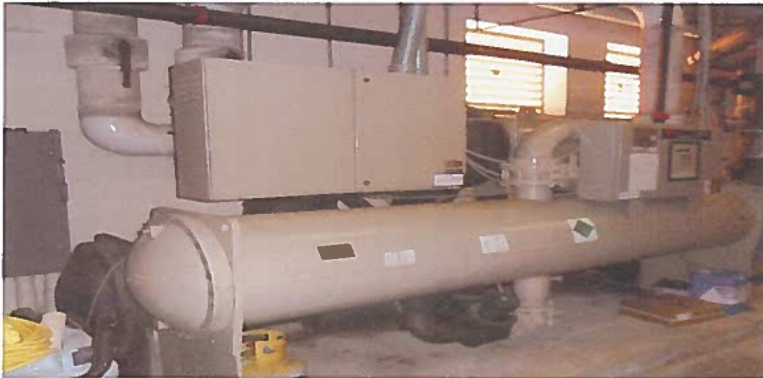
Figure 1: Kent Island High School Main Chiller
