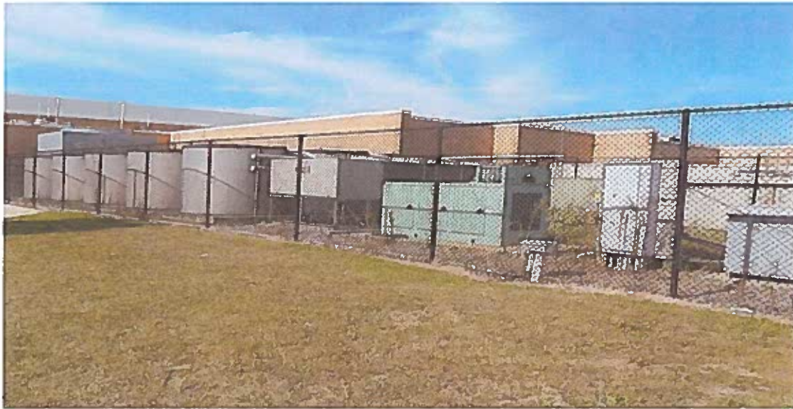
Figure 2: Kent Island High School Ice Storage Tanks
