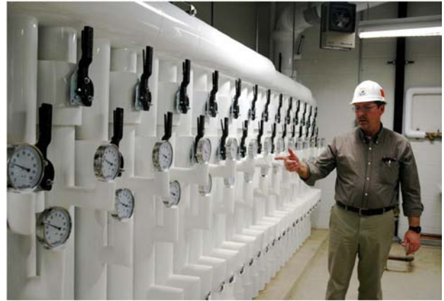
Mechanical Room, Geothermal Ground Source Heating and Cooling System St. Michael's Elementary and High, St. Michael's, Talbot County
