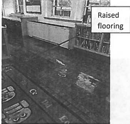
Problematic Unit Ventilator and raised floor
