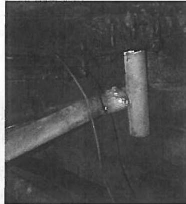
Unit Ventilator leaking pipes in crawl space
