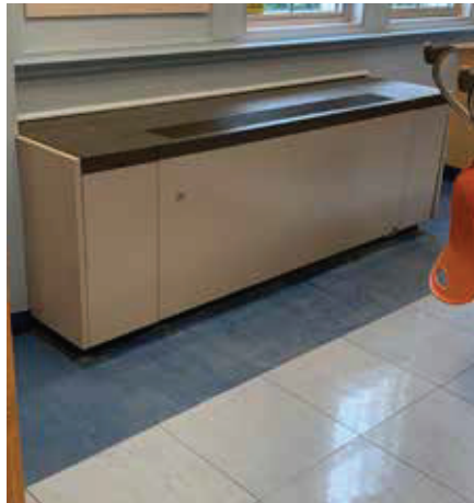
Media Center Unit Ventilator
