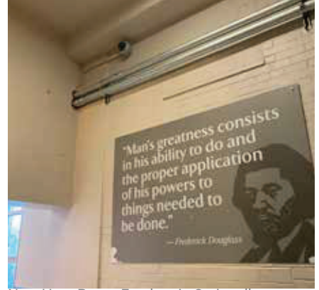
New Heat Pump Feeders in Stairwell
