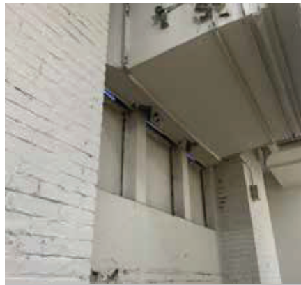
Make up Air Duct in Existing Window
