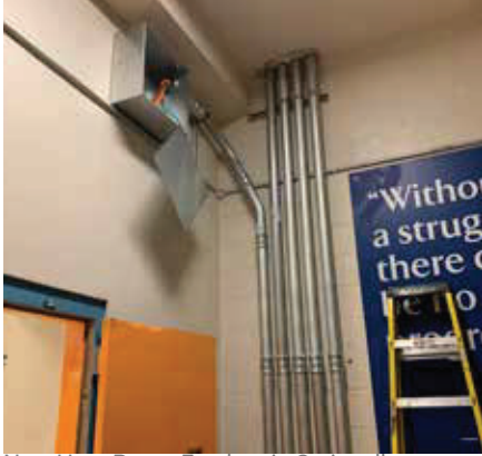
New Heat Pump Feeders in Stairwell
