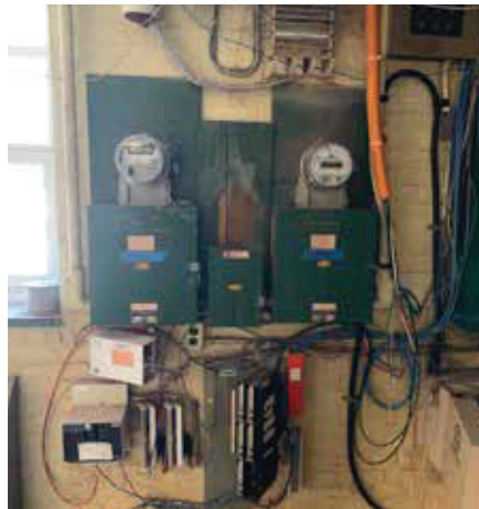
Existing BGE Metering
