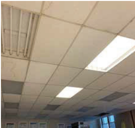
Existing Classroom Lighting
