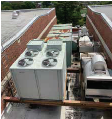
Auditorium Roof Top Unit
