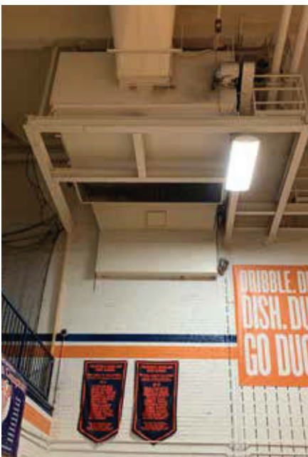
Gym Heating and Ventilation Unit
