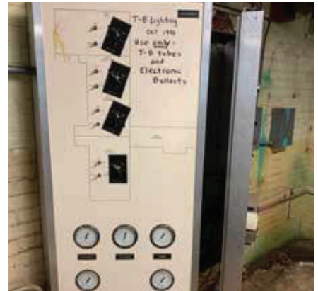
Lighting Relay Panel
