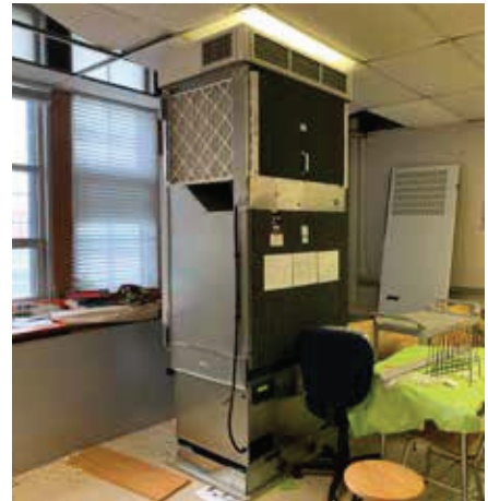
Vertical Packaged Heat Pump (Classroom)
