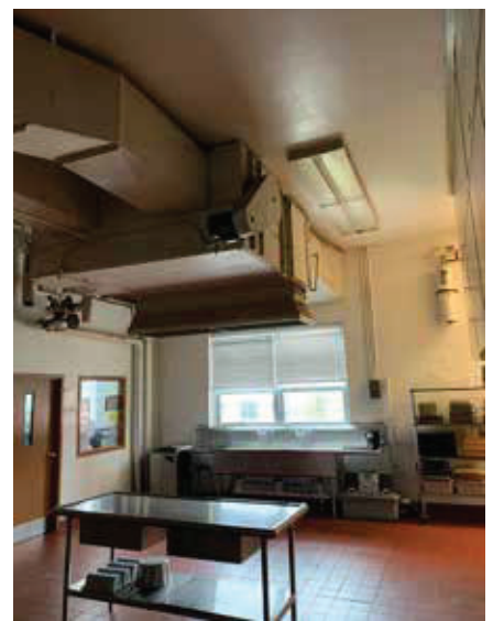
Kitchen Make up Air Unit
