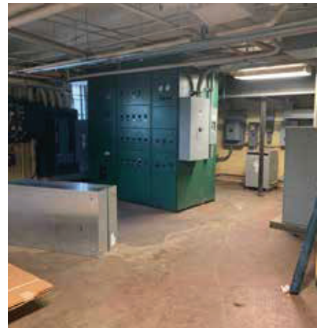
Existing 1200A Switchboard
